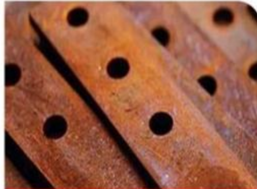
The iron parts are rusty
